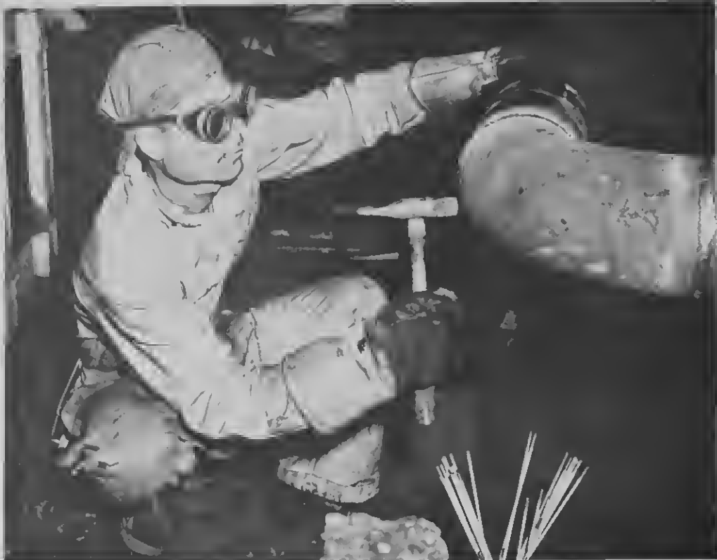
UPON completion of a welding job, excess weld is chipped off the surface. Pieces of flying weld could very easily lodge in the eye. To ward off such possible injury this employee wears protective goggles.
